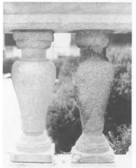
Figs. 7 a,b. The marble balusters facing the garden, top , are covered by a blackened alteration crust. The reverse sides, bottom , (facing a patio) show very little surficial alteration. Marble balusters at the Organization of American States Building, Washington, D.C.
