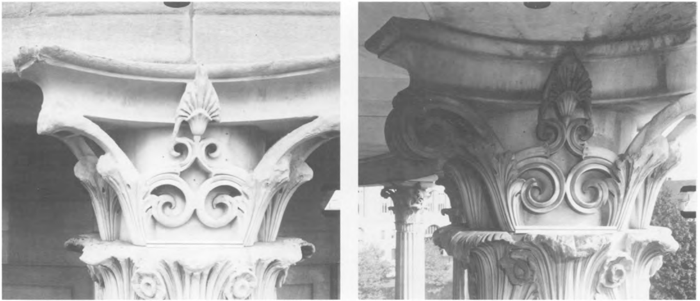
Figs. 2 a,b. Exposed volute on the column capital, left , is almost completely gone but the sheltered portion, right , still retains intricately carved details. Merchants' Exchange, Philadelphia, Pa.
